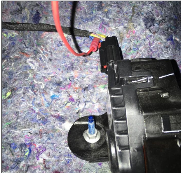
Figure 19 – TPS Signal Wires Connection
