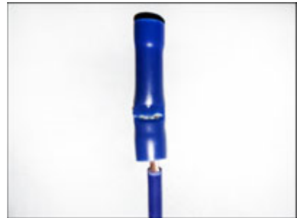
Broken Butt Connectors
