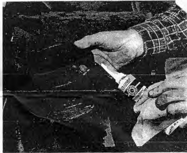
A thorough application of either Marine-Tex or windshield sealant, around the perimeter of the plastic hat assures you of a leak-tight seal. Did you remember to seal the gap between the circular dam and cowl vent lip?
