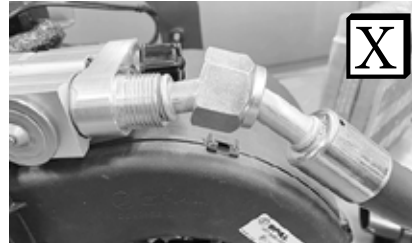
Improperly Seated O-ring Land
