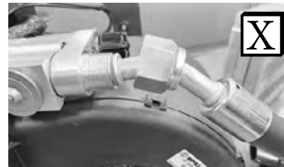
Improperly Seated O-ring Land
