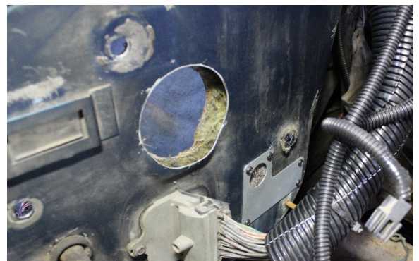
Photo 2 - 3" Hole in Firewall
